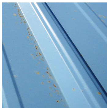
Example of red rust on the surface of a painted metal panel, caused by metal filings
